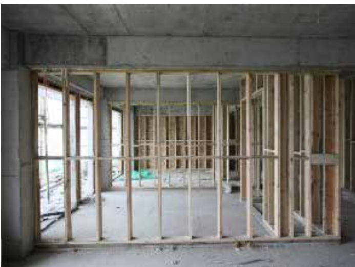
Yu Ling Long infill wall project construction showing interior partition walls and exterior infill walls in the background.
