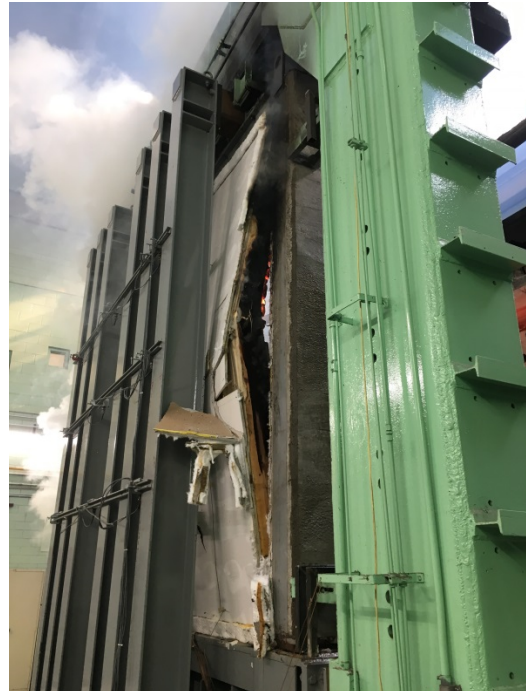
Figure 31. 2x8 NLT wall structural failure.
