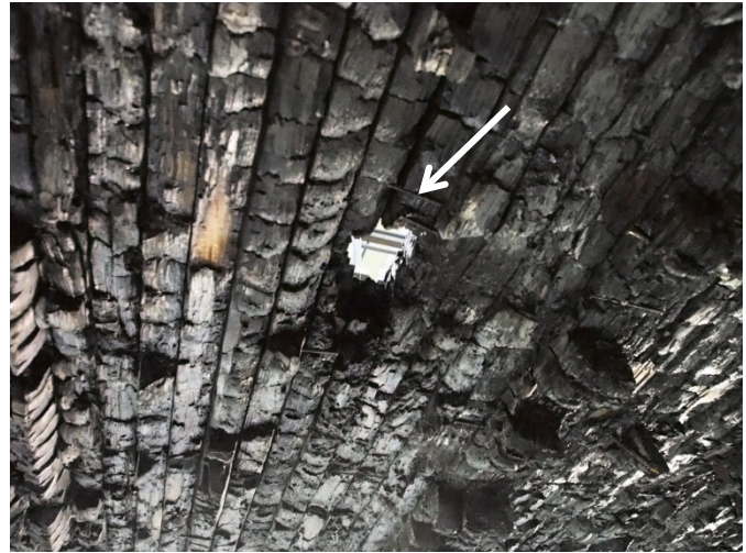
Figure 42. 2x6 NLT floor burn-through after test.
