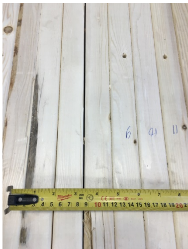
Figure 49. Gap between NLT boards.
