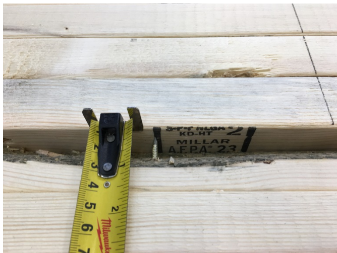
Figure 51. Gap due to wane.
