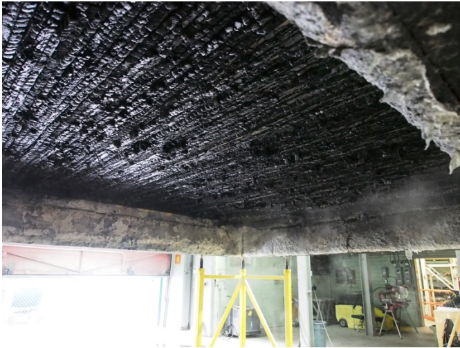
Figure 41. 2x6 NLT floor condition of exposed surface after test.
