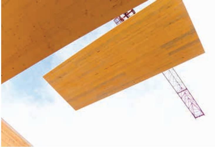
Cross-laminated timber installed during construction of the Earth Sciences Building at the University of British Columbia | Photo: KK Law
