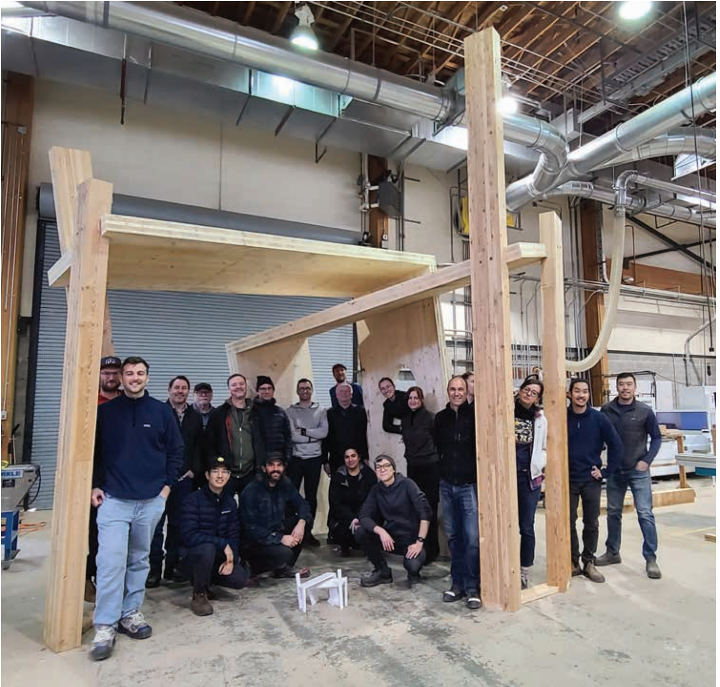
Program participants proudly pose with CLT and glulam pavilion designed, fabricated, and built throughout the three-day workshop | Photo: UBC Centre for Advanced Wood Processing
